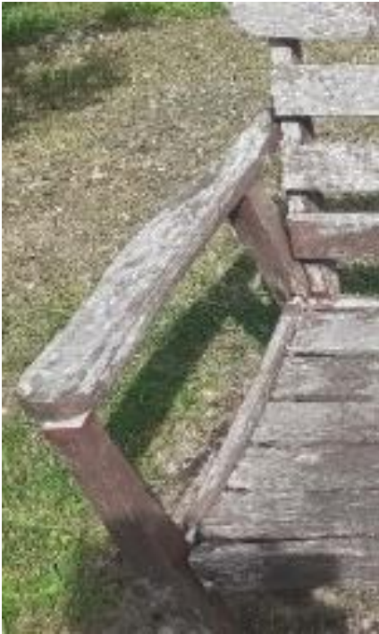
2b. cracking of wood and loose joints within the assembly of the bench.
